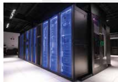
US based data center located in Chattanooga, TN
